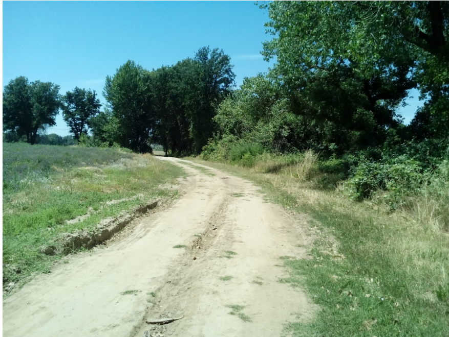
Exhibit 1 – NC2B from eastern end looking west, 15’-20’ wide, 640 feet long (Department of Regional Parks, June 2017)
