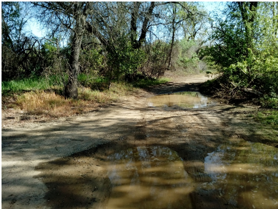
Exhibit 2 –NC2B western end, 17’ wide at intersection with NC1B and NC2 (Department of Regional Parks, March 2016)
