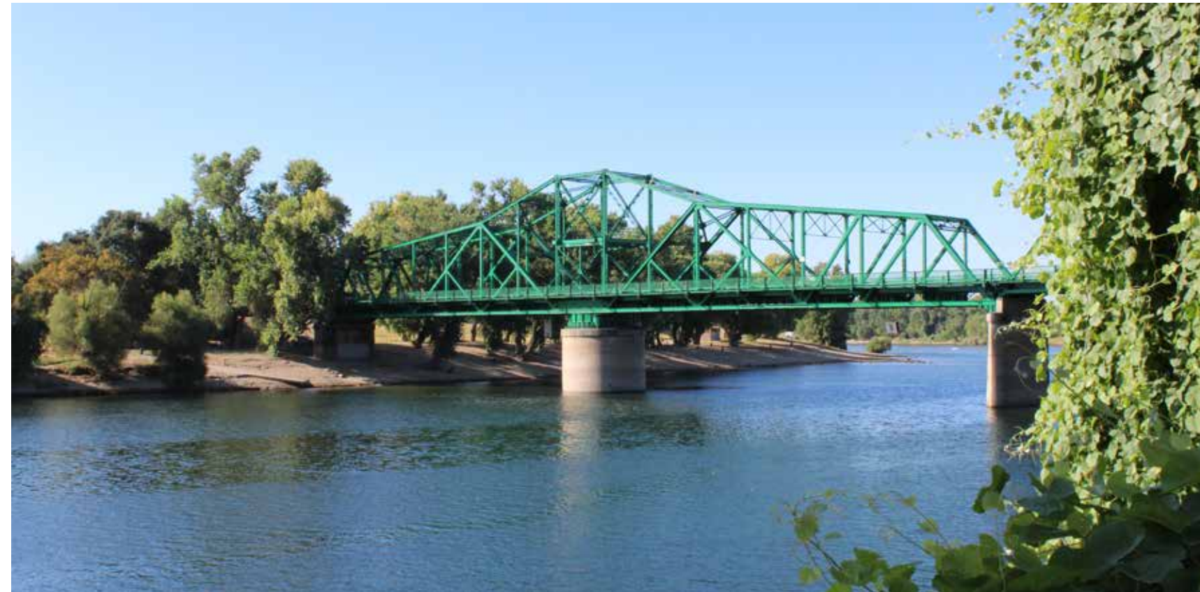
The Jibboom Street Bridge in the Discovery Park Area. Photo Credit: MIG
