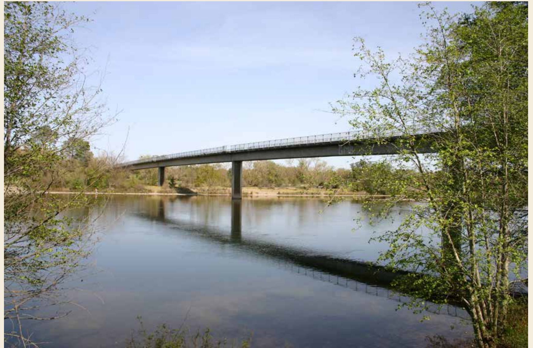
The Harold Richey Memorial Bicycle Bridge in the Arden Bar and River Bend Park Areas. Photo Credit: Regional Parks
