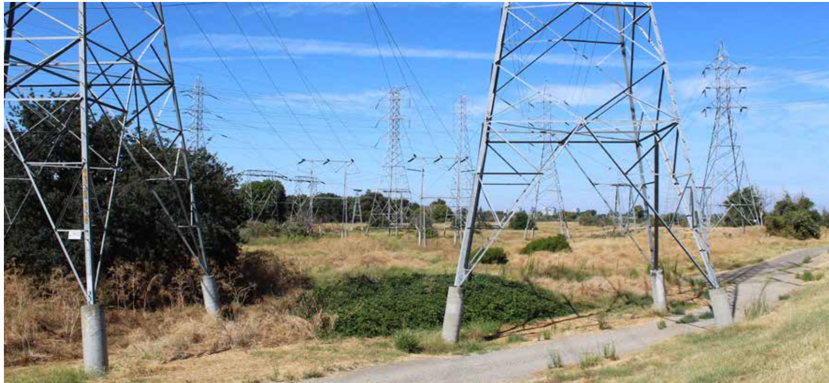
Electrical power transmission towers in the Cal Expo Area. Photo Credit: MIG
