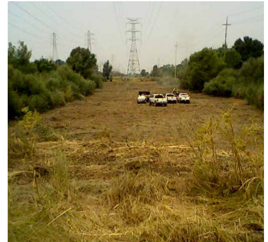
Vegetation clearing activities under WAPA powerlines in the Cal Expo Area. Photo Credit: Regional Parks
